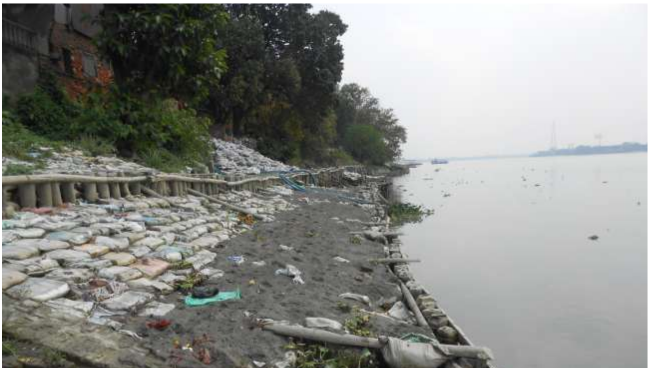
Plate 128 – Sand filled bags used for protecting river banks , Naihati Municipality, 22°53'35.80"N 88°24'40.54"E
