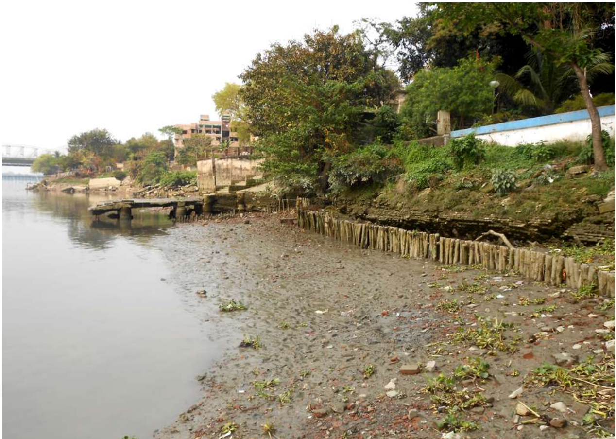
Plate 130 – Bank erosion observed in Ariadaha area , Kamarhati Municipality, 22°41'18.20"N 88°21'59.24"E
