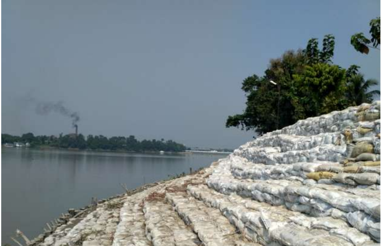
Plate 129– Sand filled Bags are used to check soil erosion near Bichali Ghat , Garulia Municipality, 22°49'24.56"N 88°21'32.91"E
