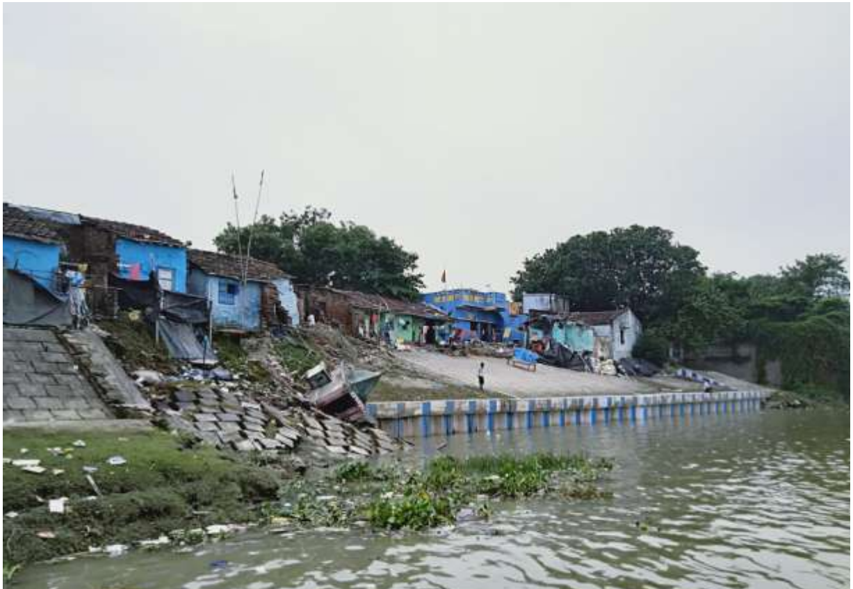
Plate 6– Embankment Breaching because of unscientific River Training Work near Shyamnagar .
